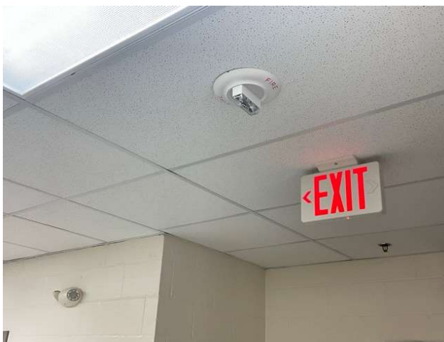
29 - FIRE ALARM DEVICES
