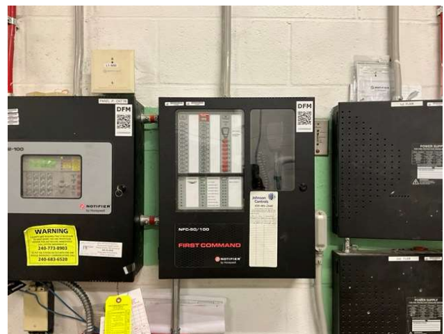
30 - FIRE ALARM PANEL
