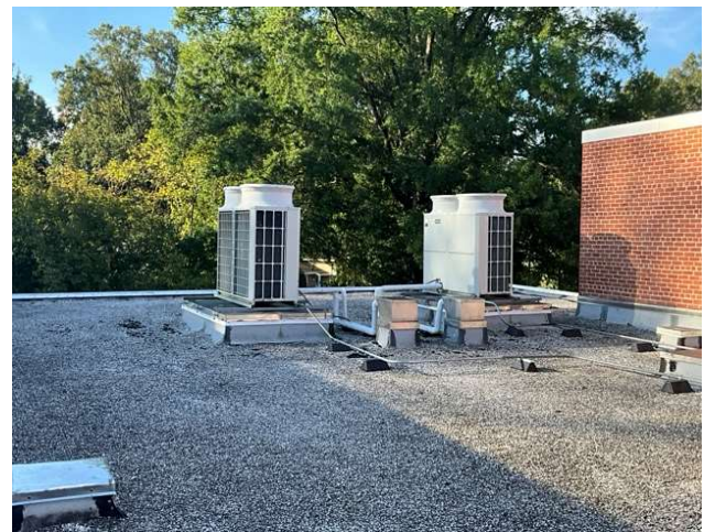
28 - SUPPLEMENTAL HVAC EQUIPMENT
