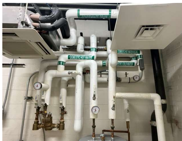
24 - DOMESTIC WATER PIPING
