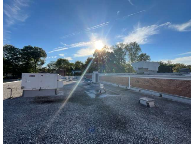
8 - ROOFTOP MECHANICAL EQUIPMENT
