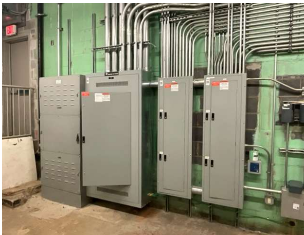
27 - MAIN ELECTRICAL ROOM
