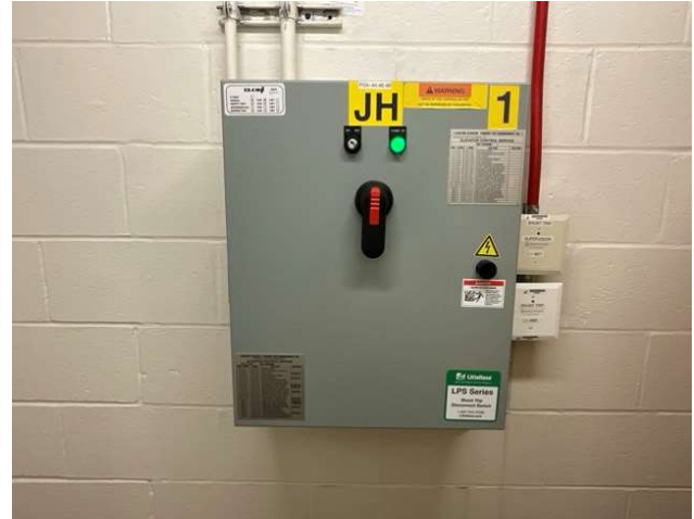
26 - ELEVATOR CAB PANEL
